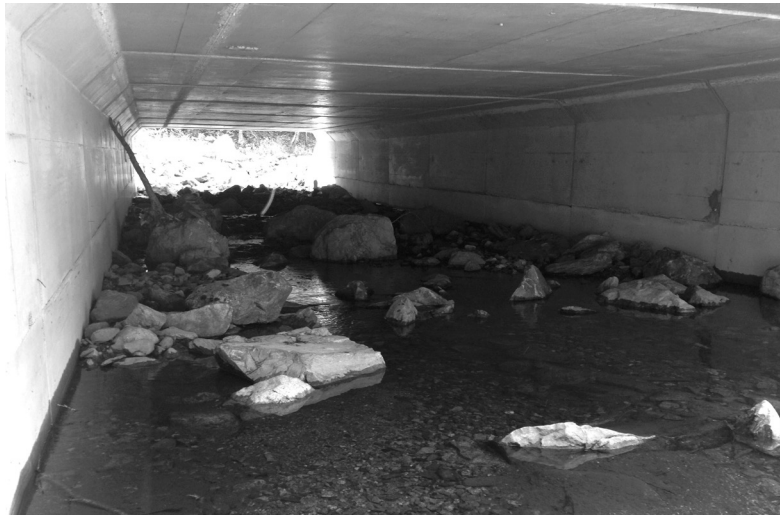
A box culvert. (Photo by MDIFW)
